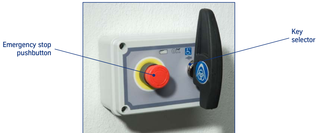
Figure 5 – Floor Call Station
